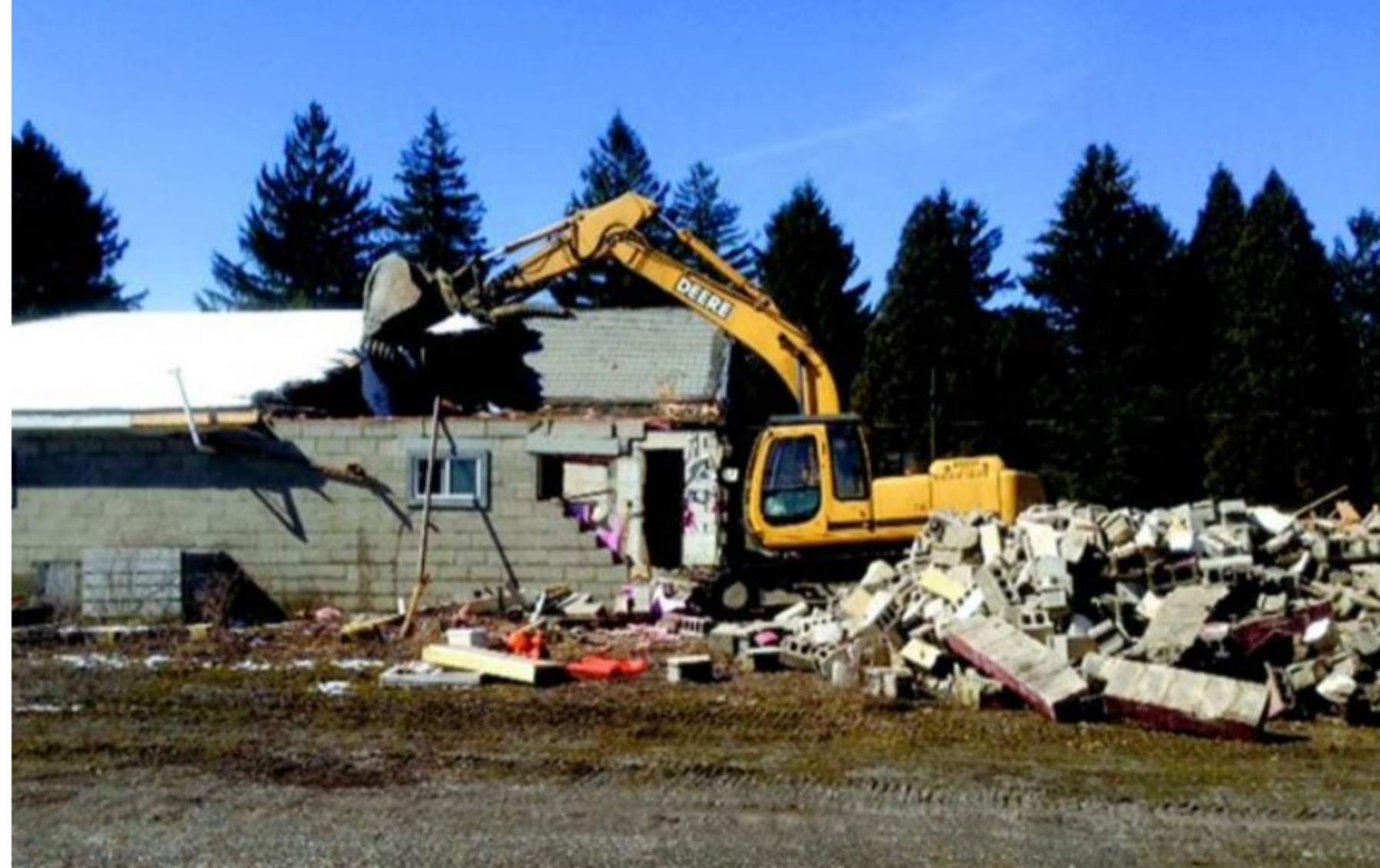
The former Neat Feat roller rink in Pine Township was recently demolished. The one-time area fun spot was closed in 1989 and had partially collapsed. The block building portion pictured was the home of the former owners Thomas and Cherie Rosak.
